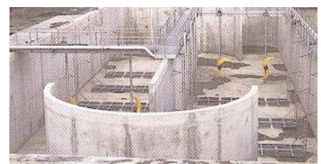
Municipal Sewage Treatment Plant (NL): 4,500 m BRANDOL®
