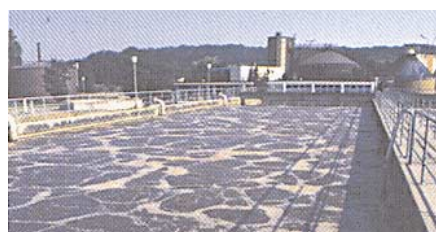
Industrial Sewage Treatment Plant Bayern (D): 1,620m BRANDOL®
