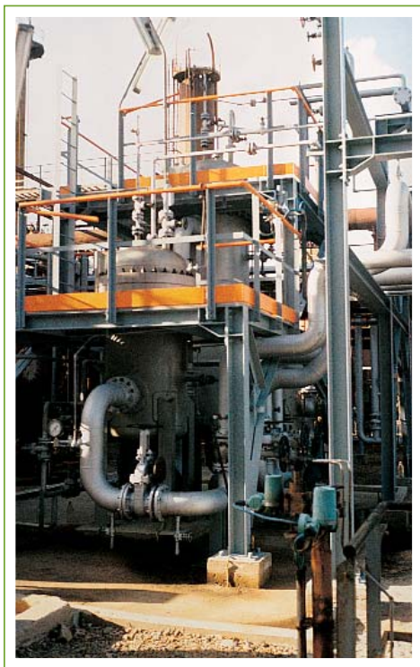
Vertical AquaSep Plus liquid/liquid coalescer system removing water from kerosene.
