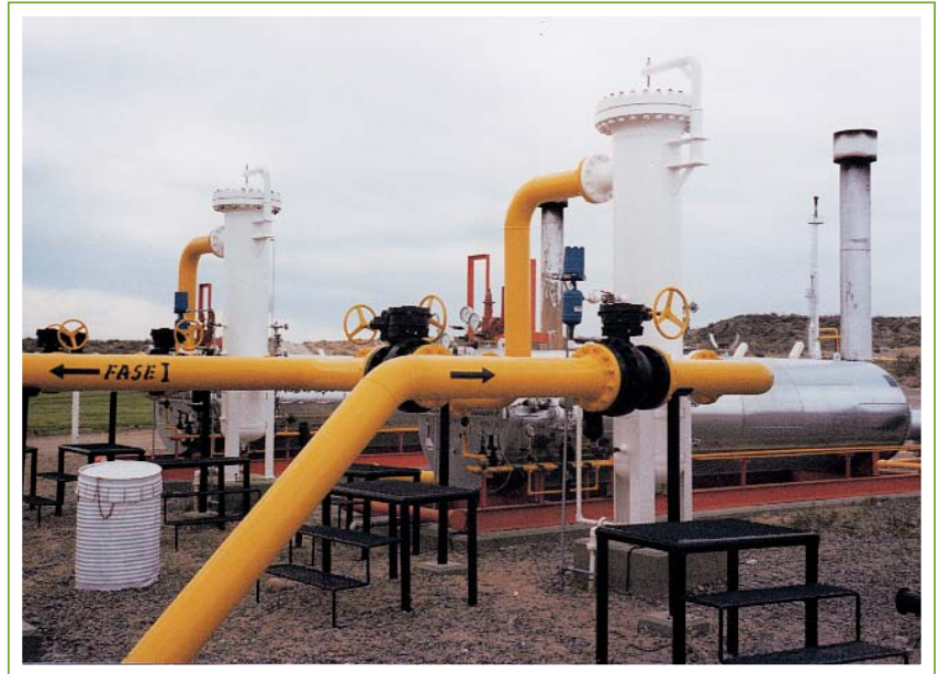
SepraSol liquid/gas coalescer system protecting a compressor.
