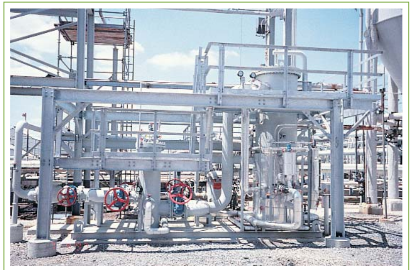
Vertical AquaSep Plus liquid/liquid coalescer system removing water from jet fuel.
