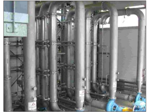
Pall Membralox Ultrafiltration Unit
