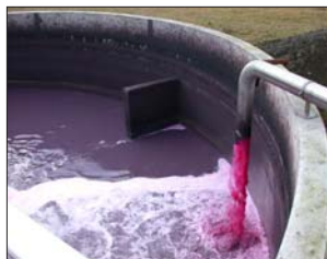
Buffer Tank Inlet
