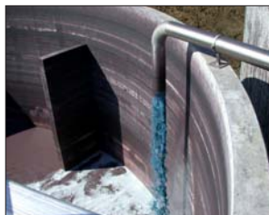
Buffer Tank Inlet
