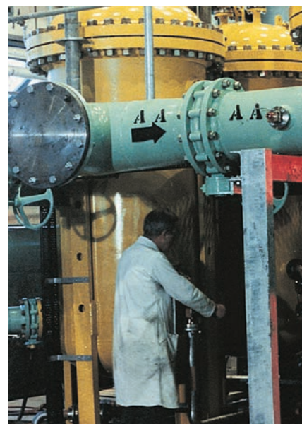
Pall's blowback filter system in operation.
