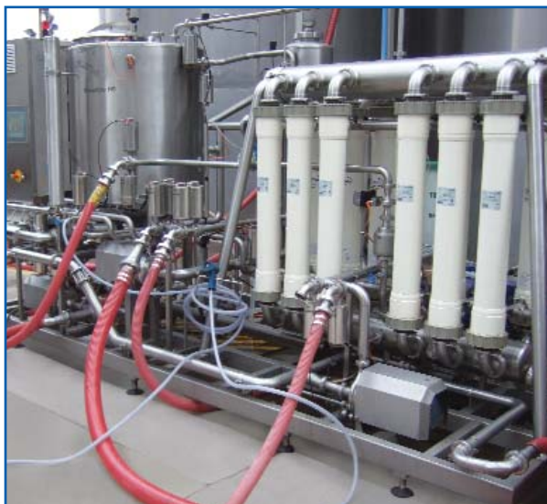
Oenoflow HS-12A System at Chilean winery
