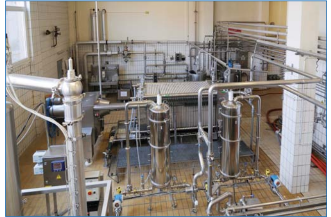
Figure 2: At one installation at a brewery, the use of SUPRApak technology saves 68% on operating costs, compared to classical sheet filtration.
