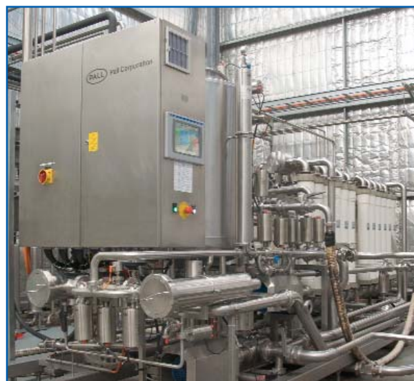
Oenoflow HS-24A System at Yalumba
