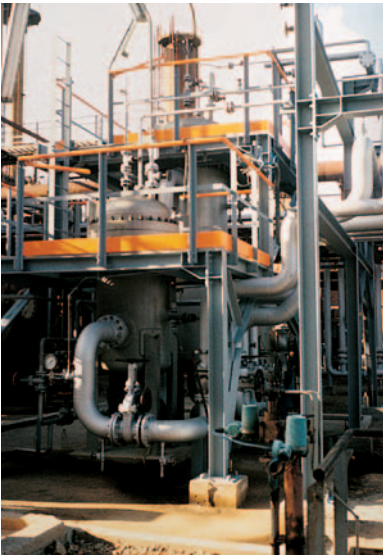
Vertical AquaSep Plus liquid/liquid coalescer system removing water from kerosene.
