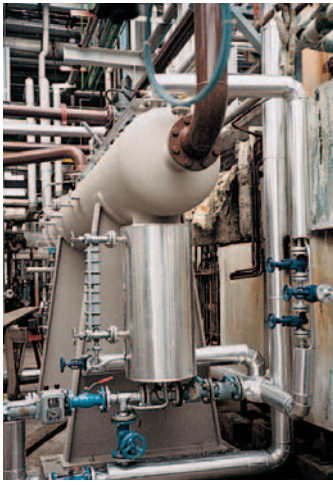
Horizontal PhaseSep liquid/liquid coalescer system removing caustic from gasoline.
