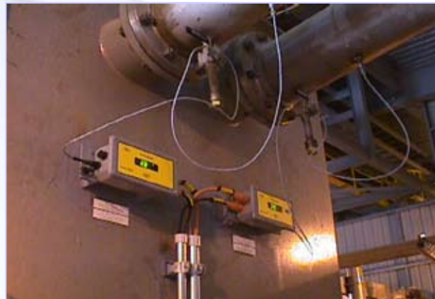
Pall WS03 Water Sensors installed on SAG Mill Lube Oil Return Lines
