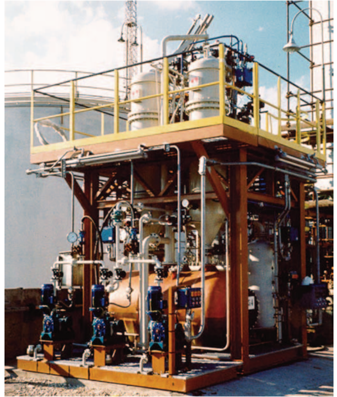
Pall backwash filtration system
