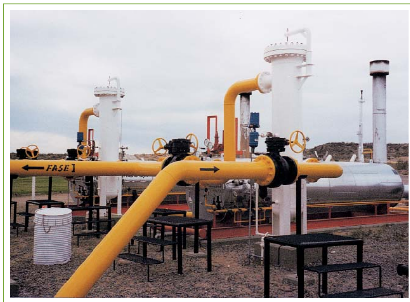
SeptraSol liquid/gas coalescer system protecting a compressor.
