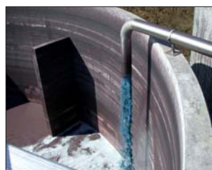
Buffer Tank Inlet
