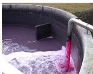
Buffer Tank Inlet
