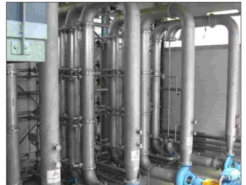
Pall Membralox Ultrafiltration Unit
