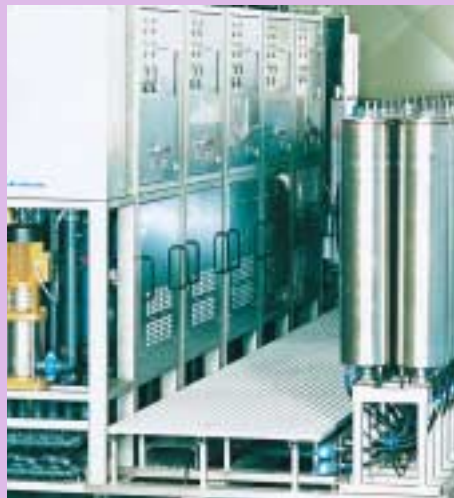
Trailer mount leachate processing system
