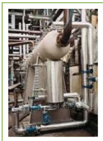
Installed PhaseSep system shown with insulated glycerin boot
