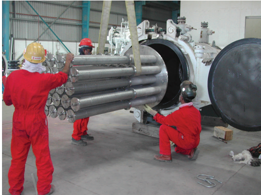
Installation of Pall's internals within the same vessel
