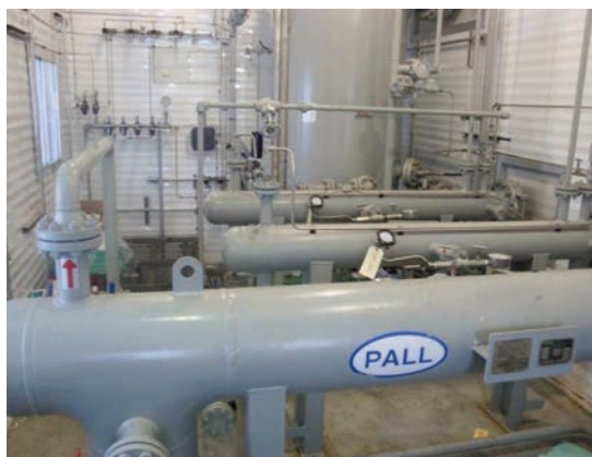
Figure 11: Overview of the Pall coalescer assembly with coalescer (forefront) and duty-standby pre-filters (background)
