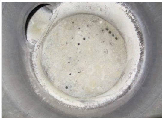
Figure 1: Salt deposits in de-ethanizer reboiler top tubesheet before (left) and after (right) cleaning (by courtesy of Crew Energy Inc.)
