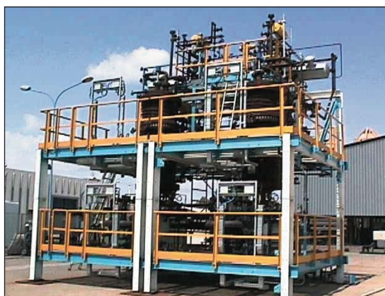
Figure 10: RFCC Slurry Oil Filter System – European Case Study #1
