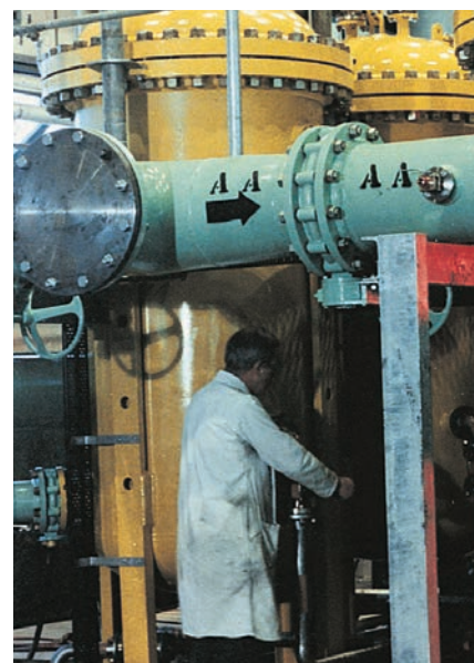
Pall's blowback filter system in operation.
