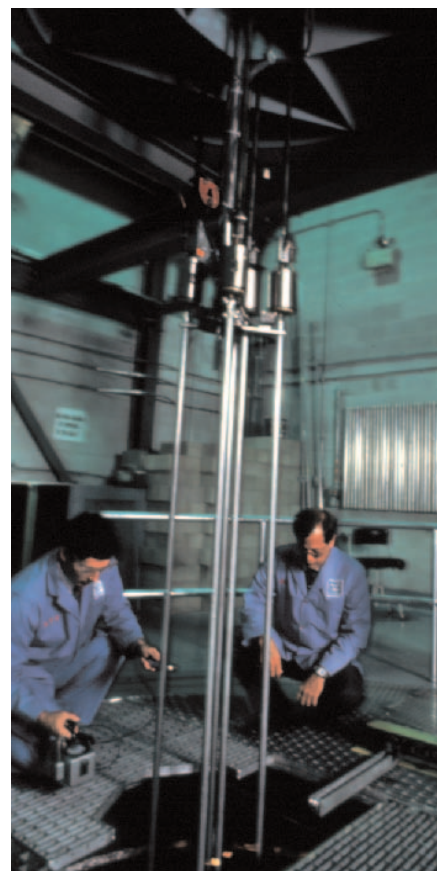
Coolant Water Filtration at a Nuclear Plant
