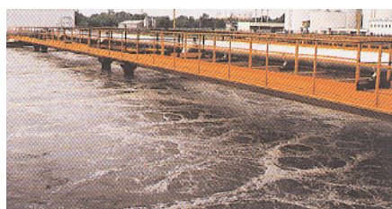
Municipal Sewage Treatment Plant Warsaw (PL): 25,900 m BRANDOL®
