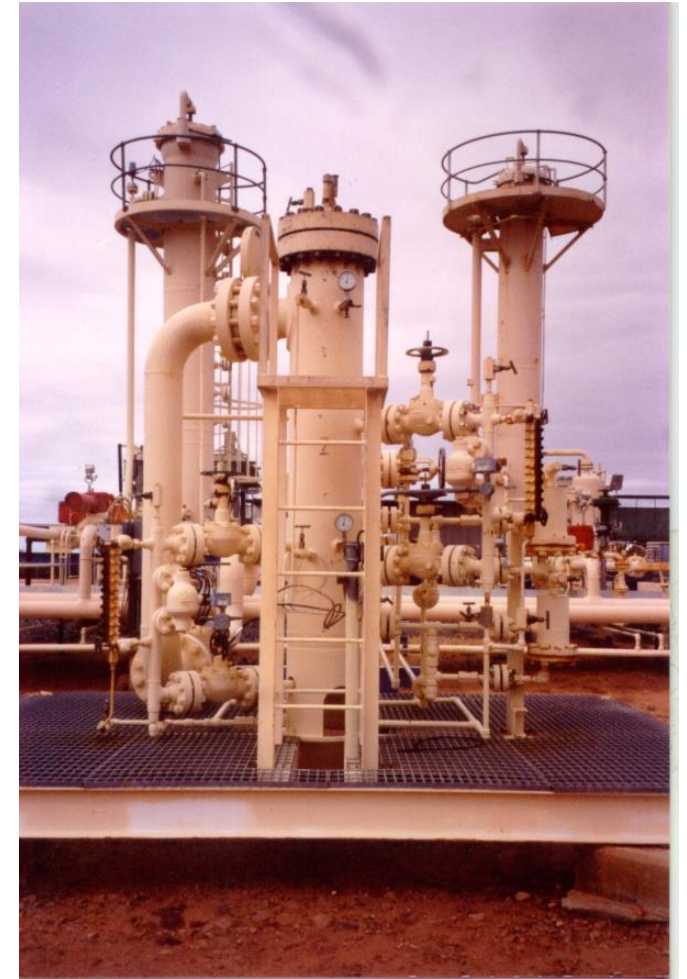
L/G Coalescer on outlet gas NT, Central Australia
