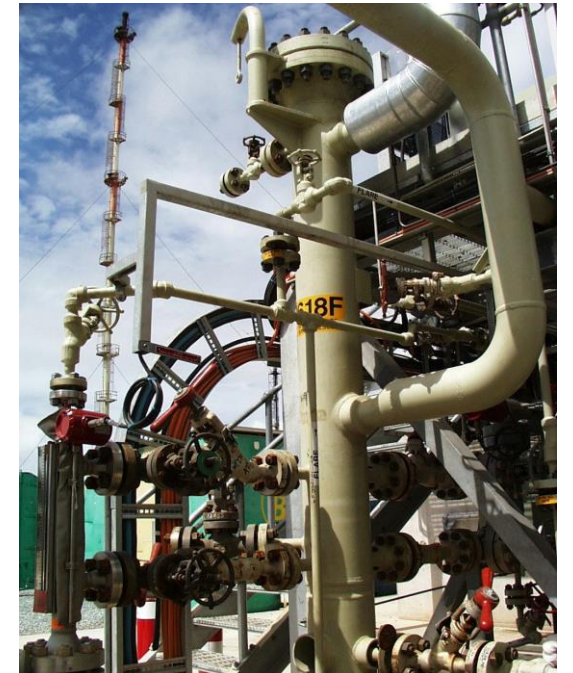
H 2 Compressor, Qld, Australia
