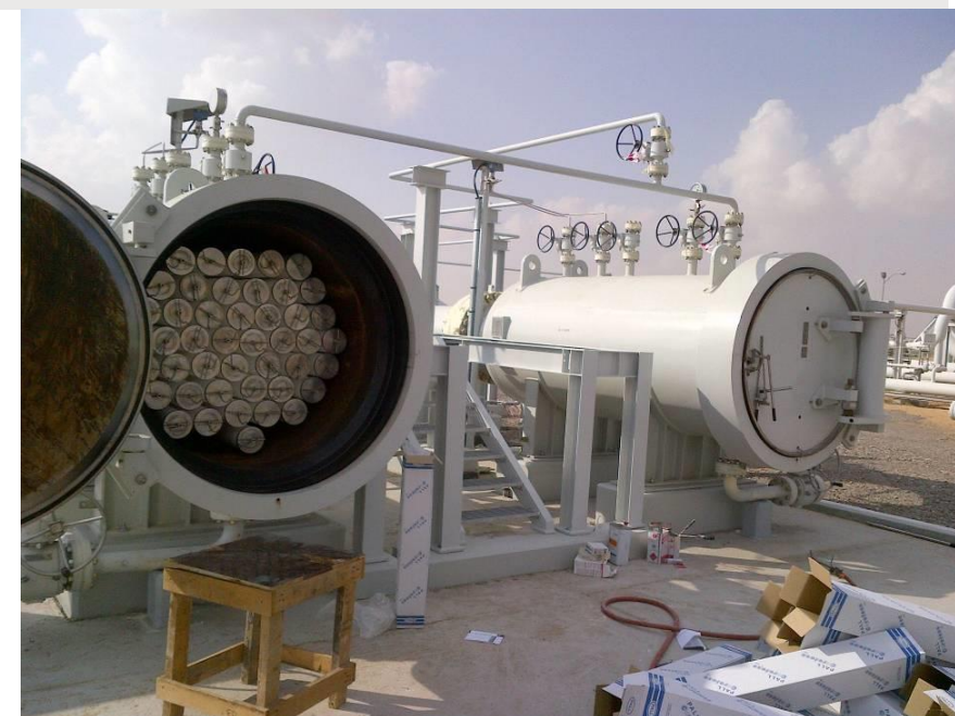
#600 Coreless Filter, 36" NB Pipeline, 700 MMscfd, 6 MPaG
