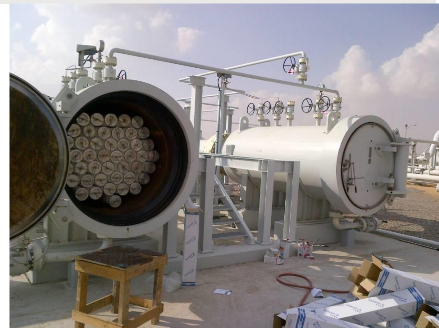
#600 Coreless Filter, UAE 36" NB Pipeline, 700 mmscfd, 60 bar g
