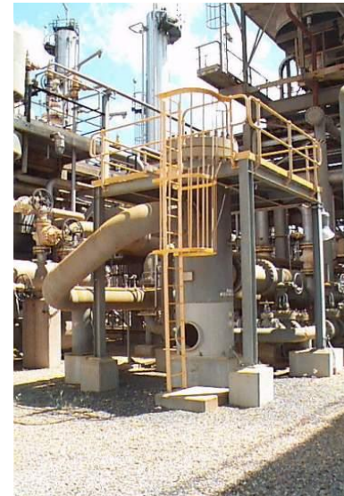
Post Drier Dust Filter
