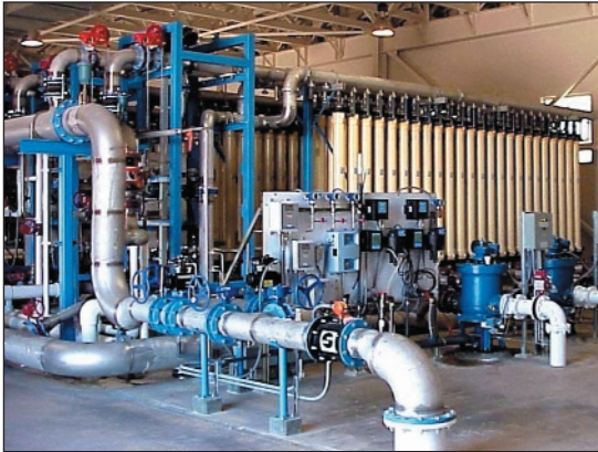
Figure 1 – 2 mgd Pall Microfiltration System at Fountain Hills Sanitary District.
