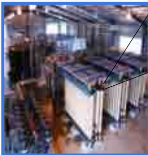
Pall's MF-RO Water Treatment System
