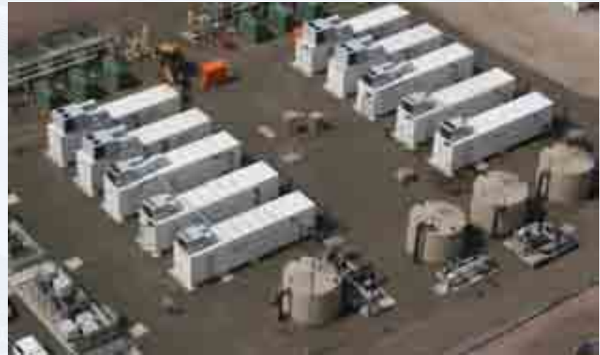
Pall Aria™ Mobile Water Systems recently installed in Queensland, Australia for Coal Seam Methane Gas Production
