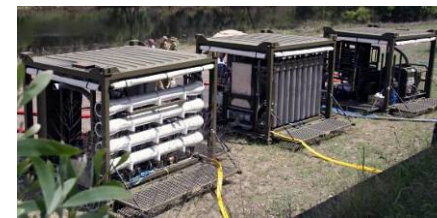
Water Treatment Systems
