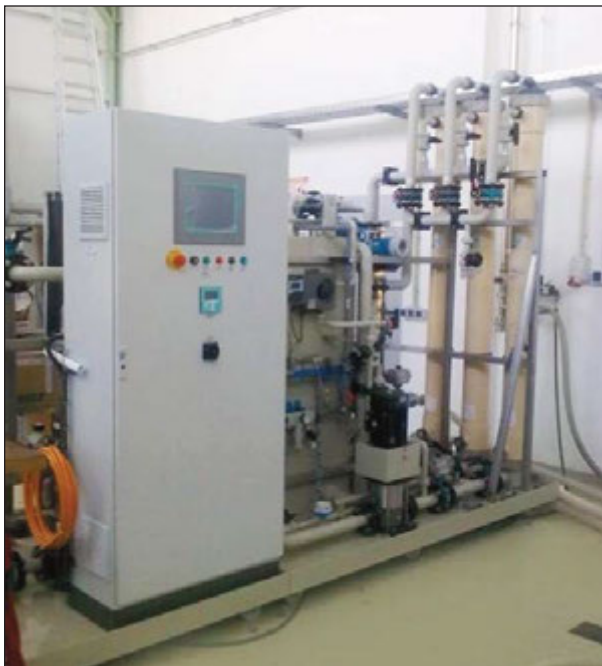
Figure 6: Pall Aria™ A1 Membrane system
