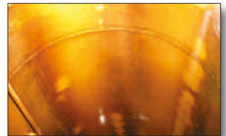
Filter housing internals coated with varnish
